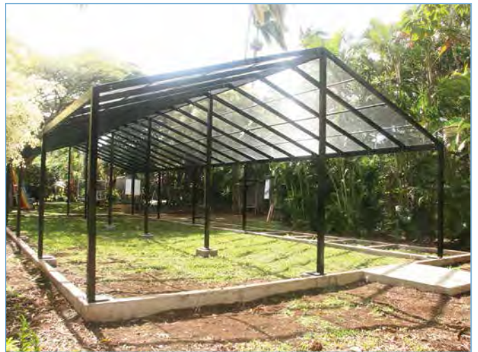
Post and beam aviary - 30'W x 75'D x 15'H, framework only with wire roof panels
