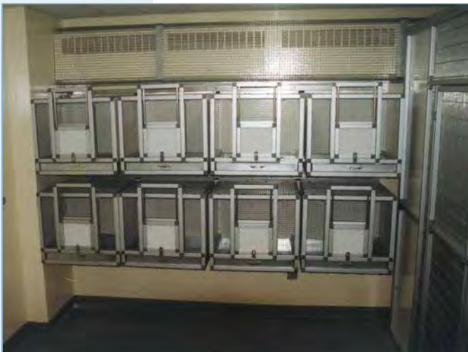
Wall mounted holding cages
