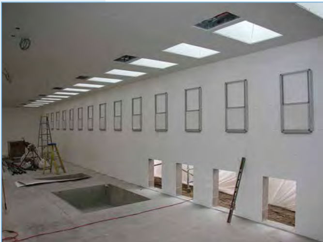
DENVER ZOO - bird propagation building, wall mounted guillotine doors, before cages were installed
