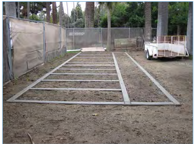
FRESNO ZOO - typical 6" wide level concrete curbs for setting panels with a natural cage bottom
