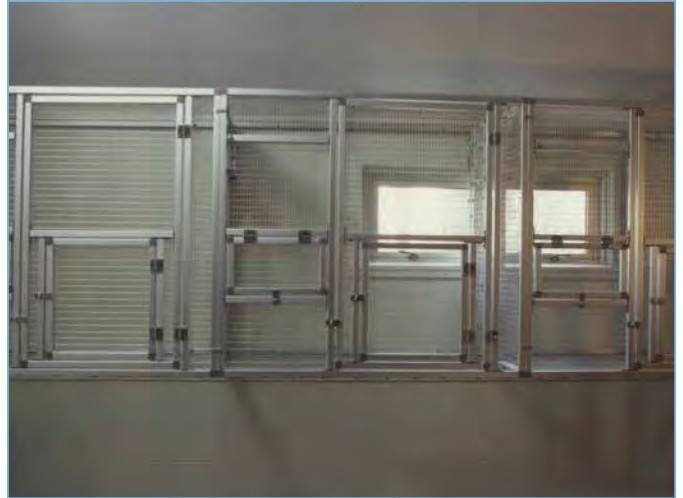
ROGER WILLIAMS PARK ZOO - wall mounted holding units
